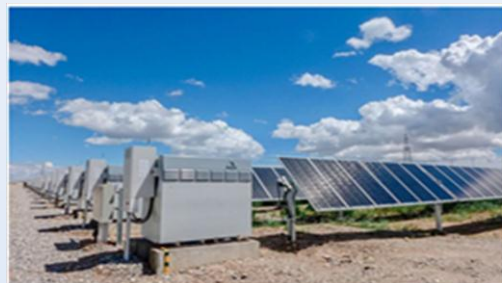
Grid-Scale solar farm with Lithium-Ion Battery storage backup.
