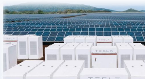
Tesla has taken the world's largest grid-scale 100 MWh energy storage project in South Australia. Installed it in a record time of 100 days.
